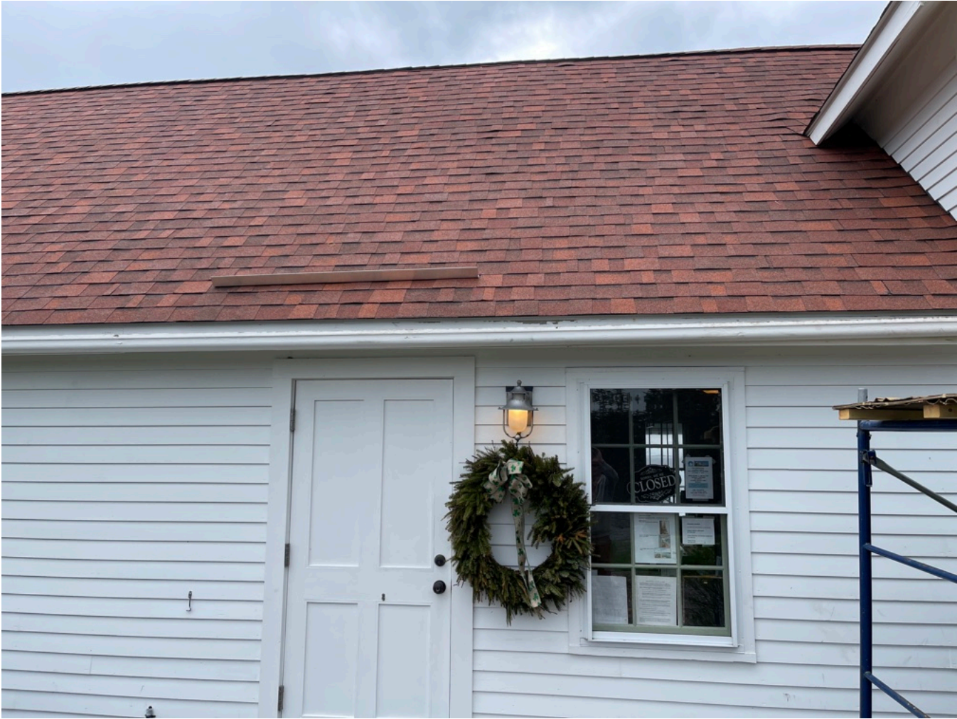
Roof Water Diverter Installed over main entrance to add to weatherstripping of front door.
